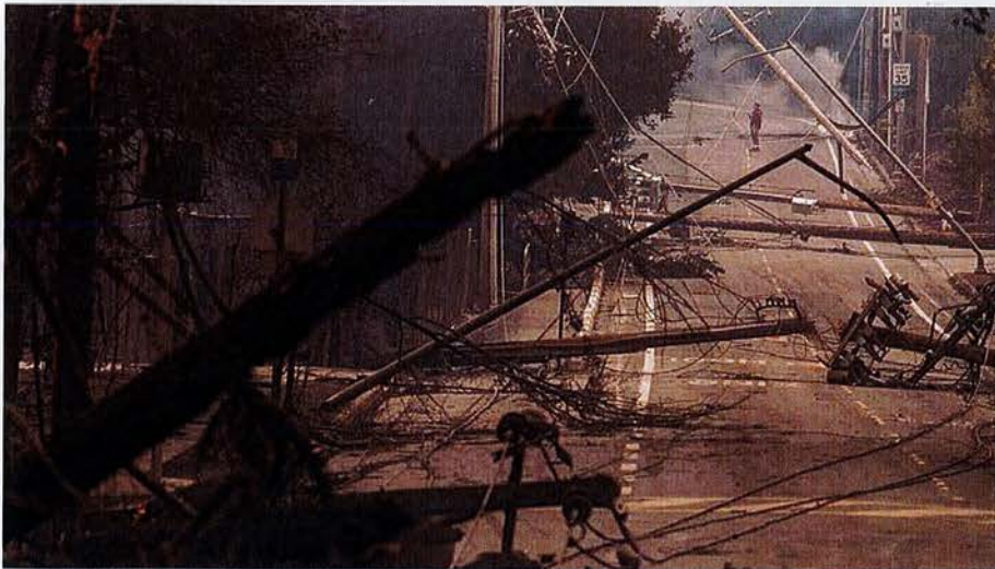
Downed power poles and lines in 2017 Tubbs Fire Photo by LA Times
